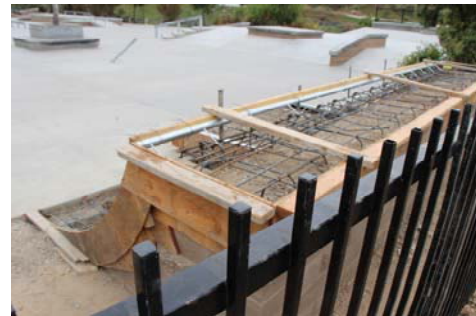
One of several ramps under construction at Black Mountain Ranch Skate Park.
